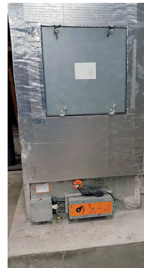
Fire damper with test switch and inspection hatch
