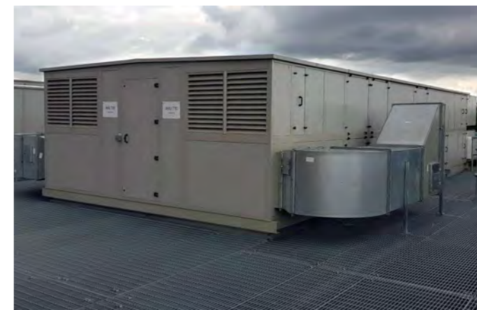
AHU formed plantroom (external)
