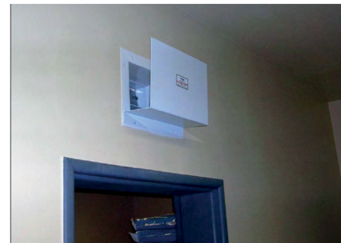
Pressure stabiliser fitted with stand-off baffle in preparation “lay up” room
