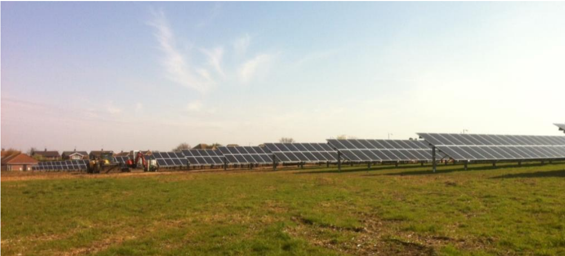
Figure 15 Photovoltaic installation at the James Paget NHSFT
