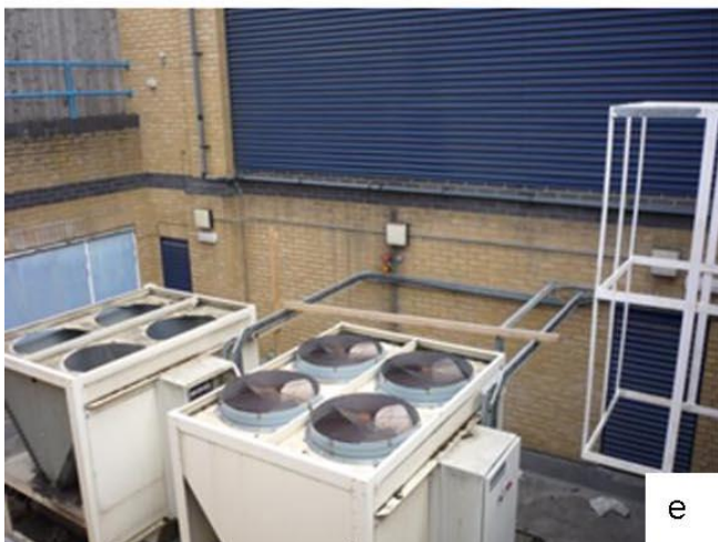
Figure 17 These pictures present examples of AC inspection findings, such as poor access for maintenance (a), incorrect use and unsuitable material of flexible ducting (b), use of wrong component parts (c) and lack of maintenance (d). Picture e presents chiller units placed directly in front of an air intake so that the heat they reject is drawn straight back into the building. Courtesy of Malcolm Thomas, Consulting Engineer.
