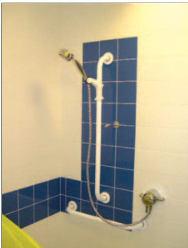
Grab rails should be fitted in bathrooms and shower areas
