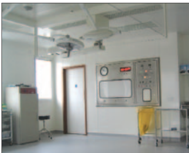
Figure 10 Theatre control panel
