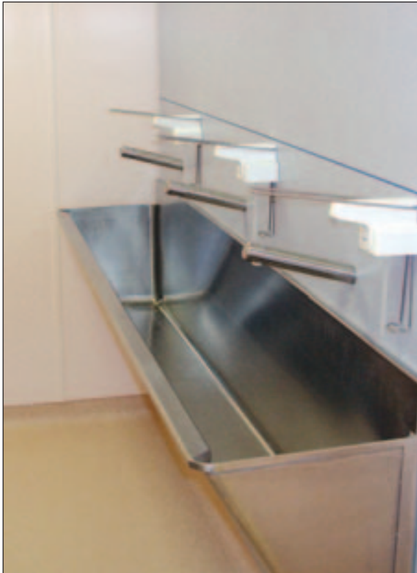
Figure 8 Scrub sink with non-touch taps
