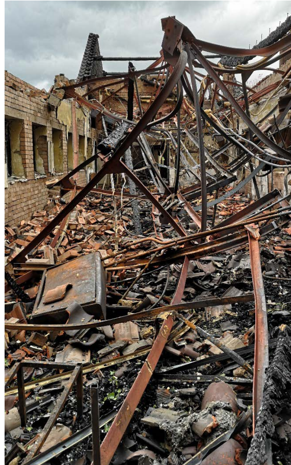
Fire damage Llanfrechfa Grange Hospital
