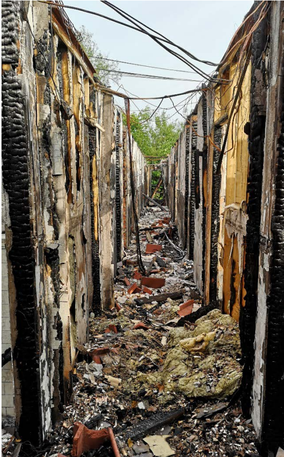
Fire damage Lansdowne Hospital
