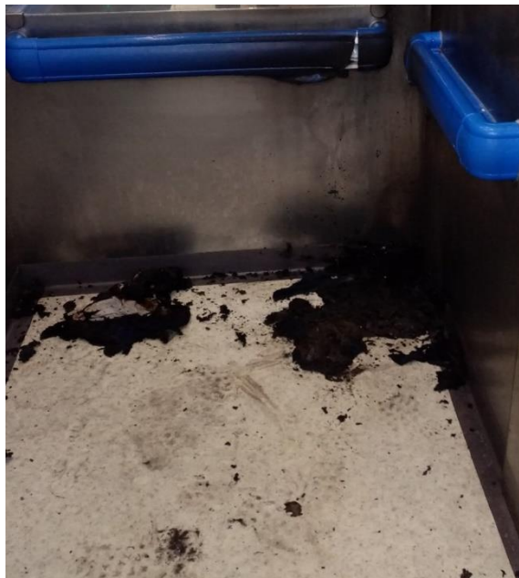
Figure 6 Example of deliberate ignition to the internal area of a lift within a Mental Health Ward
