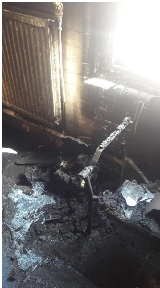
Figure 5 Example of an electrical related fire involving a small portable fridge
