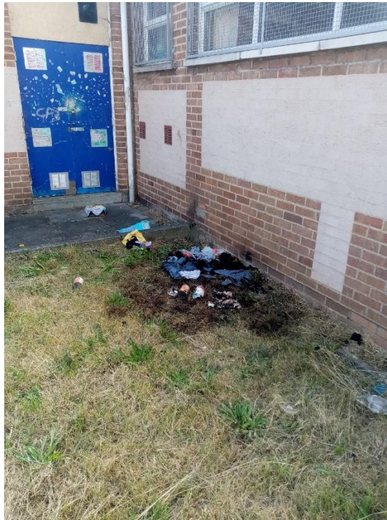
Figure 7 Example of a malicious fire incident involving deliberate fire setting to external areas, in close proximity to healthcare premises
