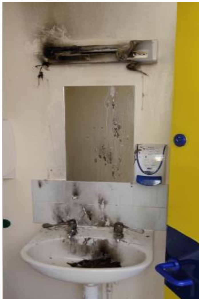
Figure 5 Example of an electrical related fire involving a lighting unit
