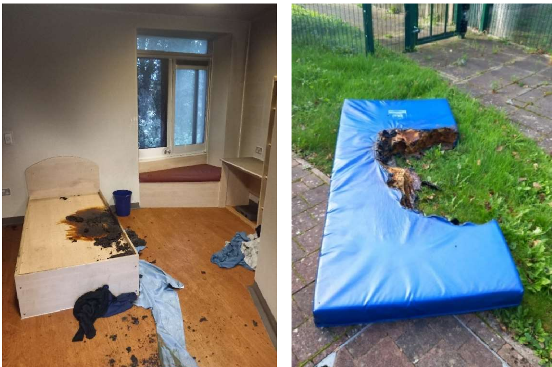
Figure 7 and 8 - Example of deliberate ignition to a bedroom within a Mental Health Ward
