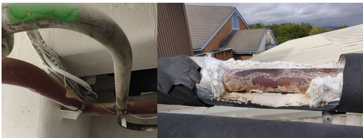
Figure 23. (left) Uninsulated steam pipe that causes significant energy waste and poses a great risk to nearby electrical installation
