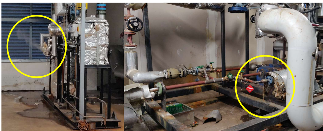
Figure 25. Steam leaks and uninsulated pipework cause both energy waste and H&S risks
