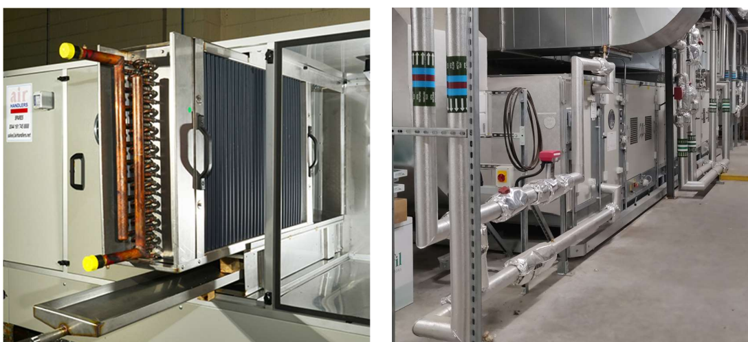
Figure 15. Heating coil of AHU
