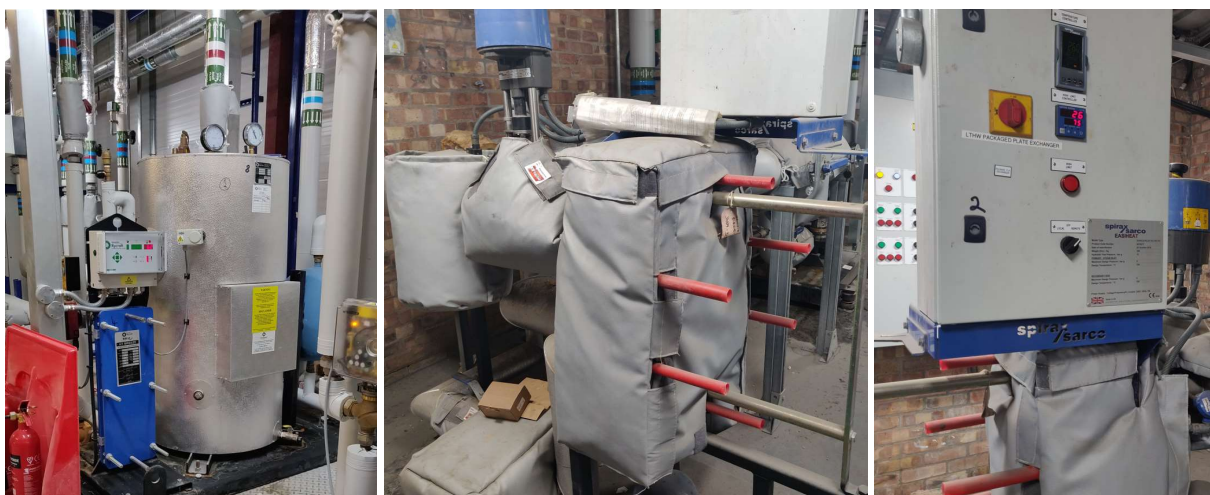
Figure 14. Heat exchanger for domestic hot water keeps the hot water vessel at 62°C (left), Steam to LTHW plate heat exchanger feeds the heating system with LTHW at 75°C (middle and right)
