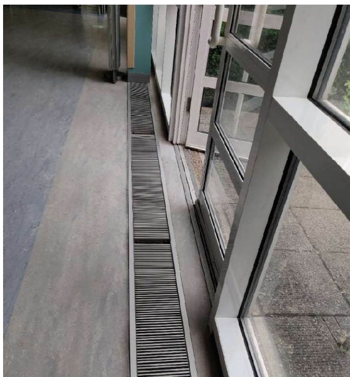
Figure 28. Perimeter heating operating with doors wedged open during winter
