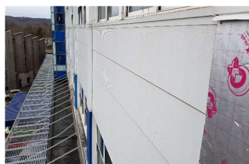
Non-compliant foam-filled spandrel panels to main facade
