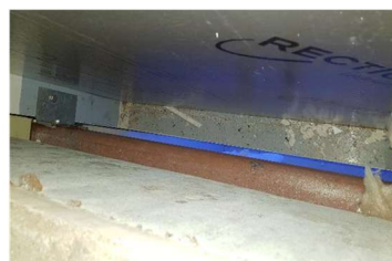
Foam insulation to rear of curtain walling and lack of fire stop between floors
