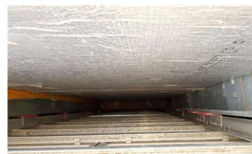
Foam insulation to flank wall and lack of cavity barriers
