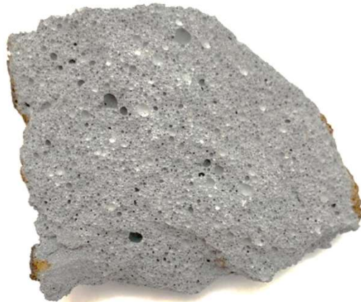
RAAC Close Up Close up of RAAC section. Note that the colour of RAAC may vary depending on the manufacturer.
