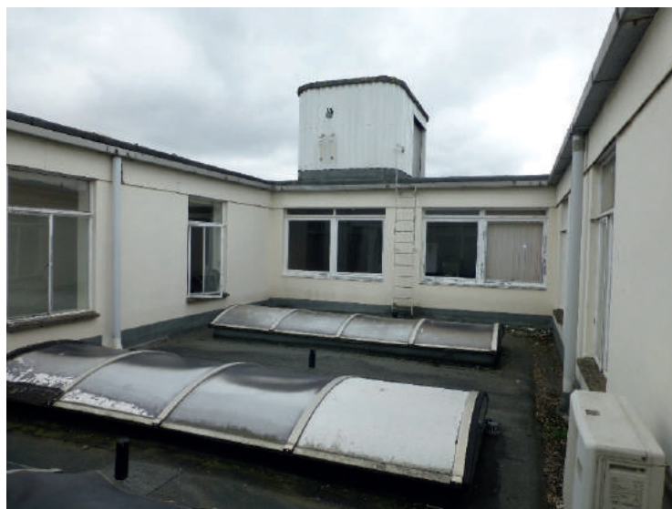
Plate 1 Enclosed single-storey building section with wooden fascia boards at the top of each wall
