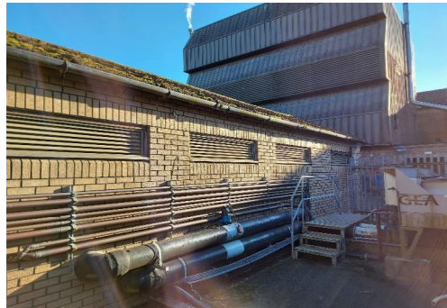
Photo 4 – Ventilation louvres in the existing building directly facing where the switch room will be constructed.
