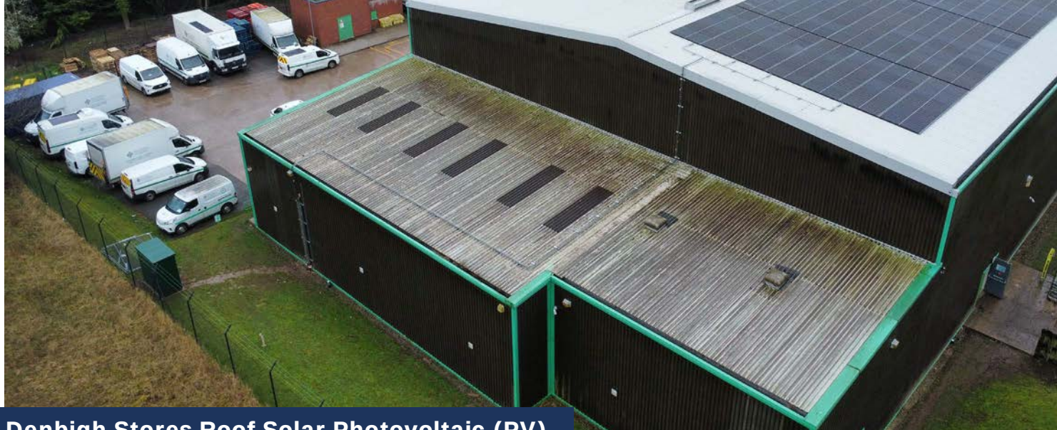
Denbigh Stores Roof Solar Photovoltaic (PV)
