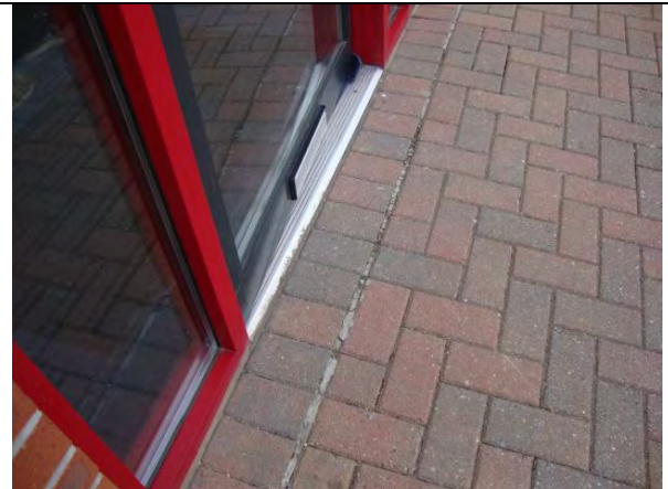
Concrete Fillet Loose
