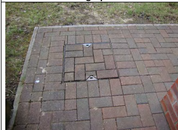
Joints to Paving Open
