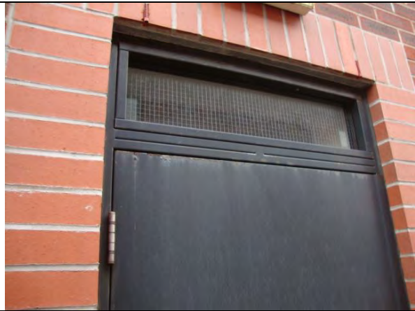
Corrosion to Door Head Photograph 57
