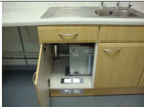
Water Cooler in Place
