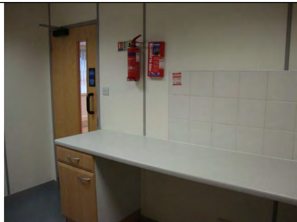
Fire Blankets in Place
