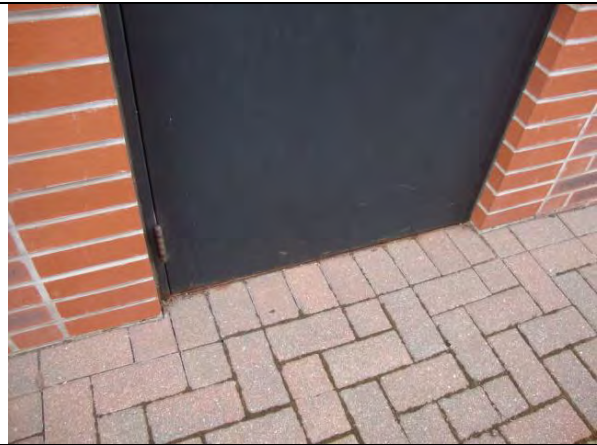
Corrosion to Door Edge Photograph 58
