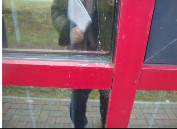
Window Frames Not Cleaned. Surfaces Soiled Photograph 56
