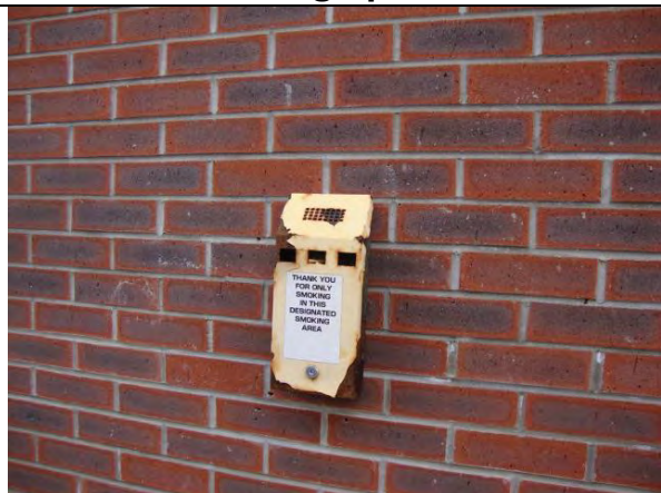
Corrosion to Ashtray Photograph 59
